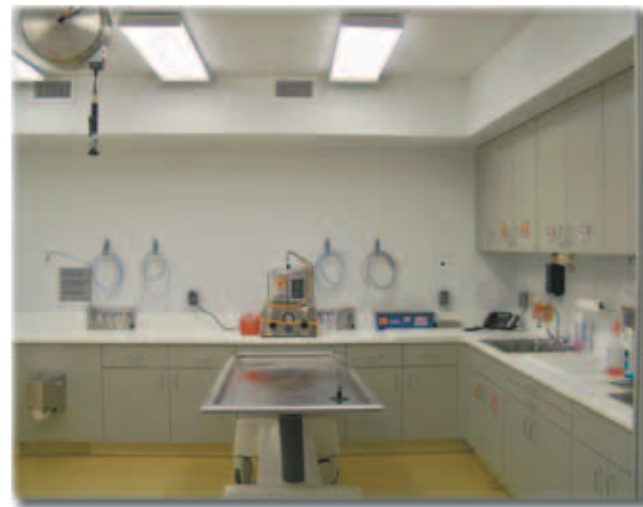
Prep room featuring DST PrepAir HVAC system
