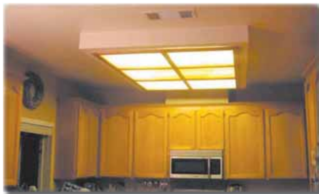
BEFORE with florescent lighting
